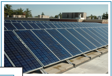
Figure 2.4 This 51kW photovoltaic system supplies approximately 6% of the electricity needs for Whitman-Hanson Regional High School, a 234,500 SF award-winning pilot project for the Massachusetts Green Schools Initiative.
